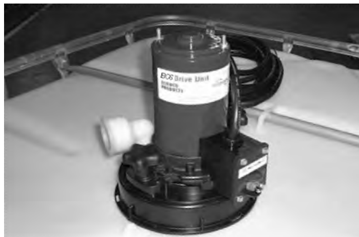
BC6 pump on cage tank.
